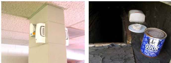
Several wall mounted aerosol deodorizers (left), and passive and aerosolized deodorizers placed within the roof top package units (right) were used in the facility. The facility spent approximately $1,100 annually on deodorizers in an attempt to “control” malodors.
