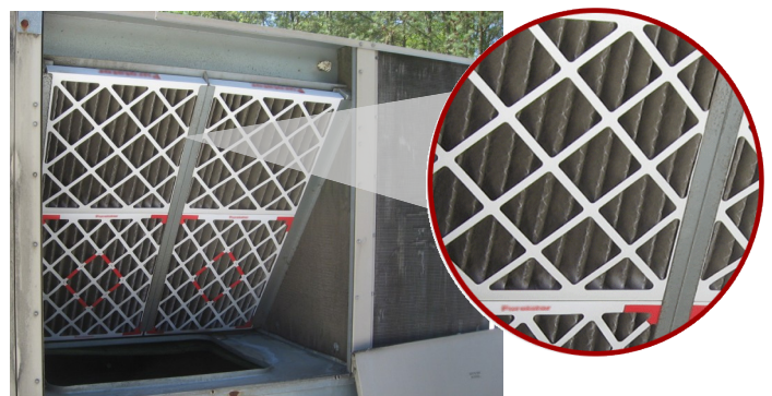
Photo of inadequate existing filtration (particulate only) within a typical roof-top package unit serving the facility. Insert shows dust-loaded competitor filter used.
